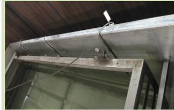
Sensors in the tank
