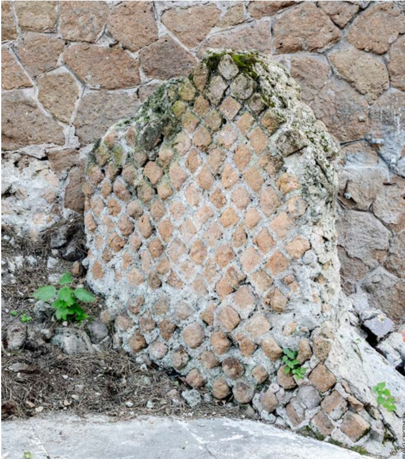
Remains of Roman opus reticulatum walls of structures believed to be tabernae (shops, workshops and commercial premises), currently visible in the building A car park.
