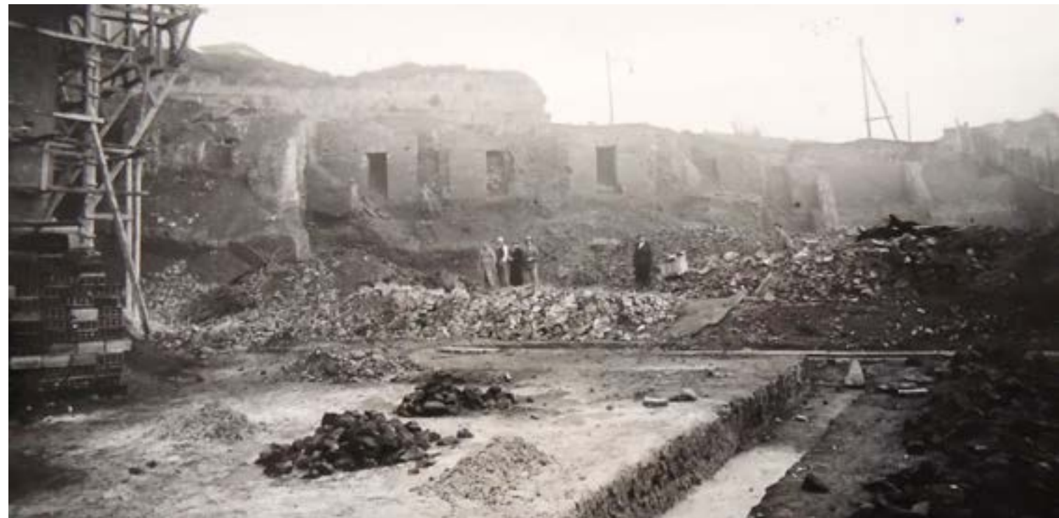
The structures that came to light in 1938 during construction of the Ministry of Italian Africa (FAO archive).
